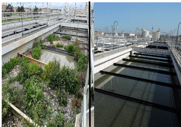
Before and after: Sediment and debris accumulation in a primary sedimentation tank resulting in compliance issues.
