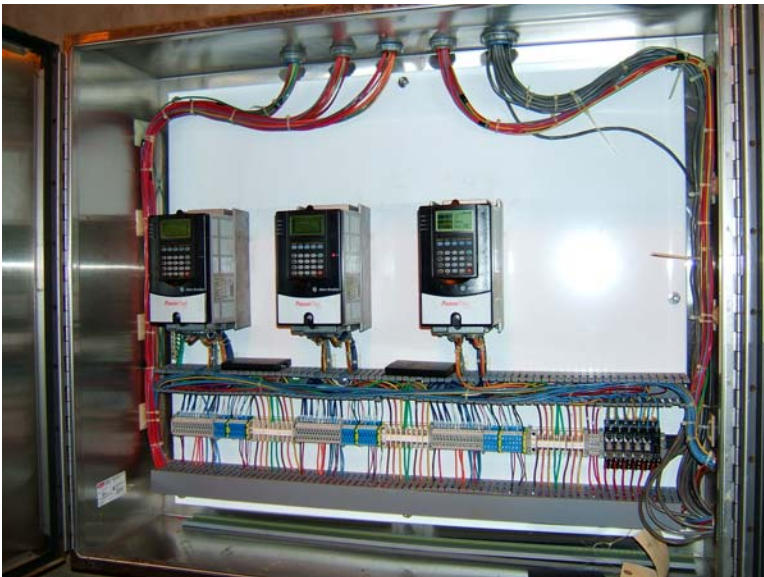
VFDs for Ferric Chloride Feed Pumps to Grit Chamber
