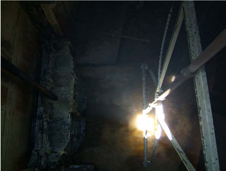
Ferric Chloride Feed Manifold at JB1
