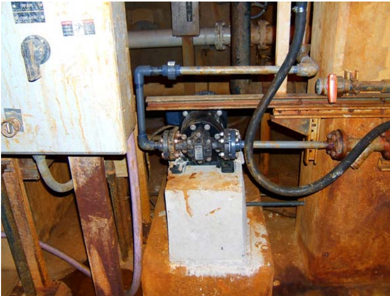
Old Ferric Chloride Feed Pumps for Grit Chamber
