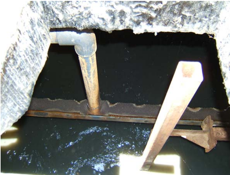
Ferric Chloride Feed Manifold at Grit Chamber
