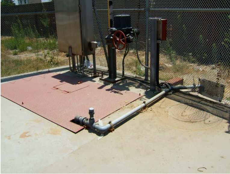
Ferric Chloride Feed Piping to JB1
