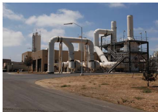
South Bay International Wastewater Treatment Plant.
