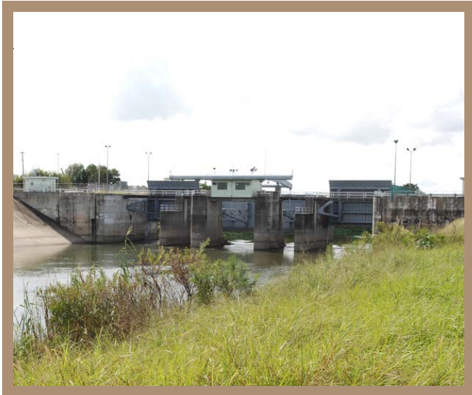
The Commission operates and maintains Retamal Diversion Dam.
