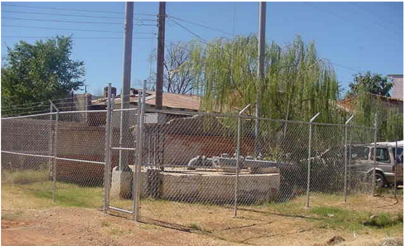
Wastewater infrastructure in Naco, Sonora
