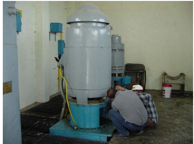
Morillo Drain pump
