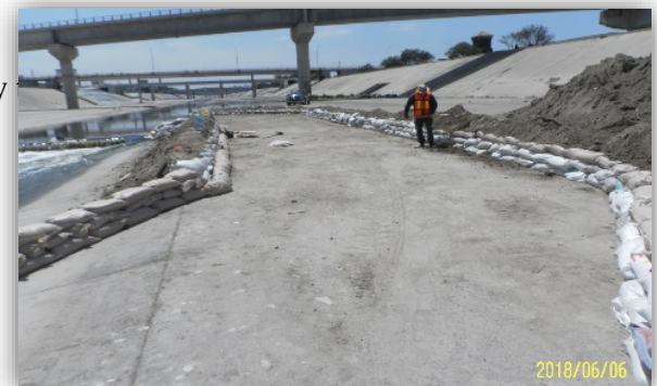
Construction of the sandbag weir in the Tijuana River channel in Mexico.
